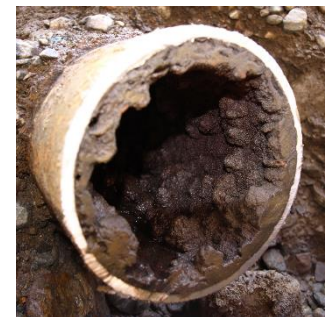
Corroded Iron Water Main
