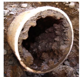
Corroded Iron Water Main
